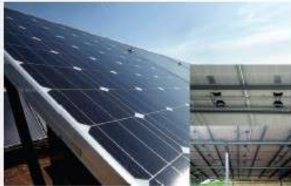
Solar panel support
